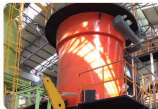
6 열매체보일러 (Thermal Boiler)
