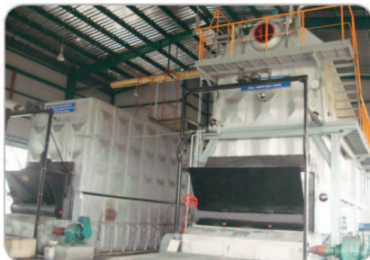
석탄보일러 Coal Fired Boiler
