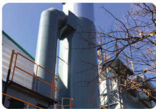
13 반건식반응기 (Semi-Dry Reactor)
